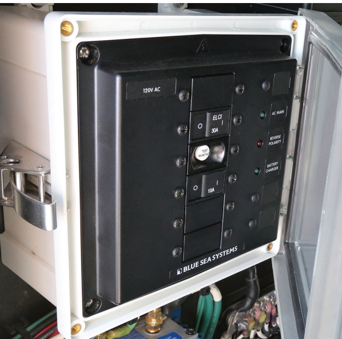
Equipment Leakage Circuit Interrupter (ELCI)
